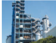
Kawasaki Plastic Chemical Recycling (KPR) plant
