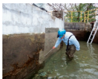
Field test of repairing material Higashinagahara (Waterway for Asahi Dam); Fixing water leaks along a wall
